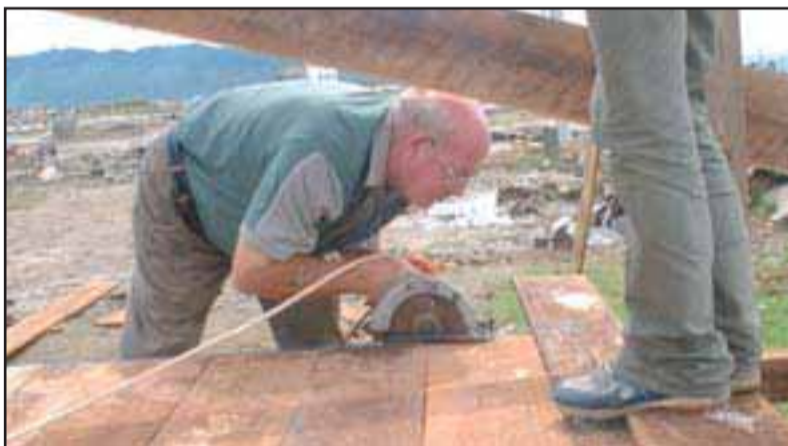
(top): Eric Doherty helps rebuild a home in Banda Aceh; (above): using a power tool - after your money helped buy a generator
